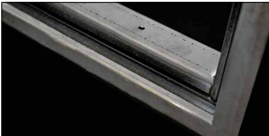
SMOKE SEAL AROUND PANEL DOOR
